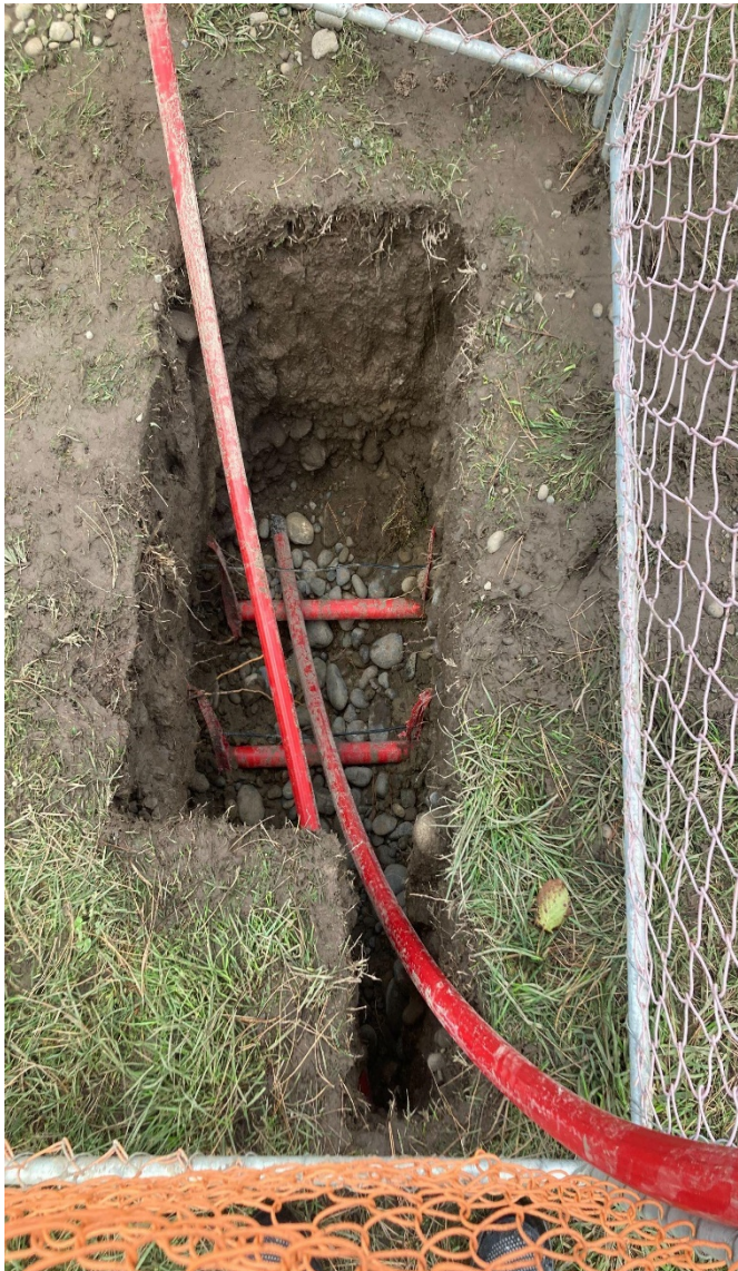
Photo six: Enable Networks - installing duct containing fibre optic cable underground. These look like single tubes but have 24 small tubes inside.
