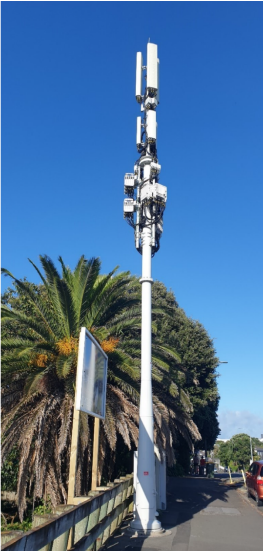
Photo two: Spark tower with 5G antenna at 448 Devon Street, New Plymouth.
