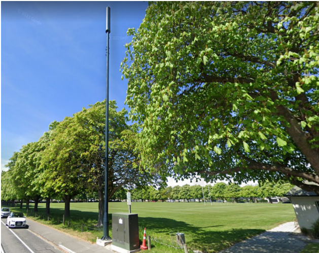
Photo one: Fortysouth pole, antenna and cabinet in road reserve adjoining 180 Innes Road, St Albans.
