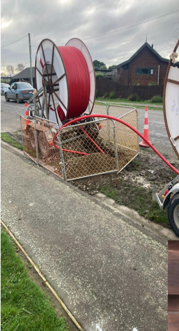
Photo seven: Enable Networks - installing duct containing fibre optic cable under the road reserve.
