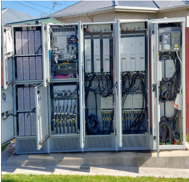
Photo five: inside of a residential roadside cabinet for a cell site.
